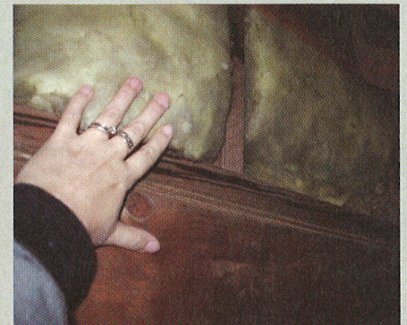
The porch roof connection has a gap in the wall sheathing.
