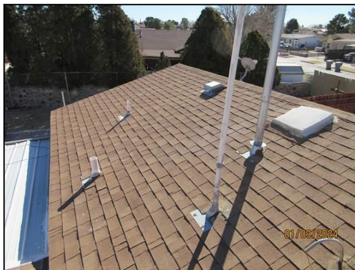
3. In the opinion of the inspector the roof...
