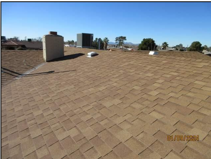
1. In the opinion of the inspector the roof...
