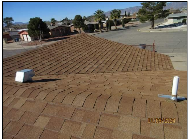
2. In the opinion of the inspector the roof...
