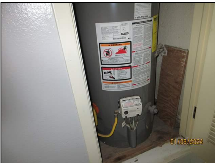
13. No plumbing recommendations are offered as...
