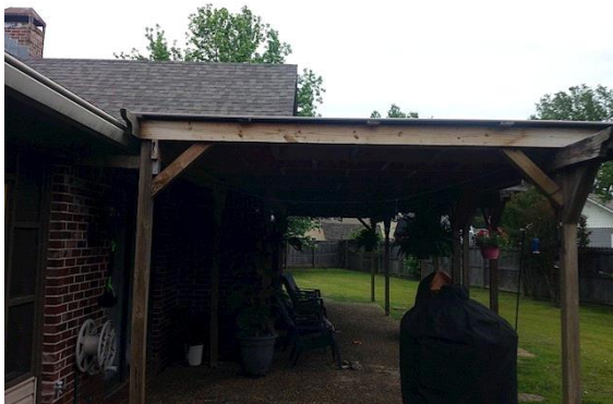
PATIO: Roof covering leaks at seams and slopes towards home
