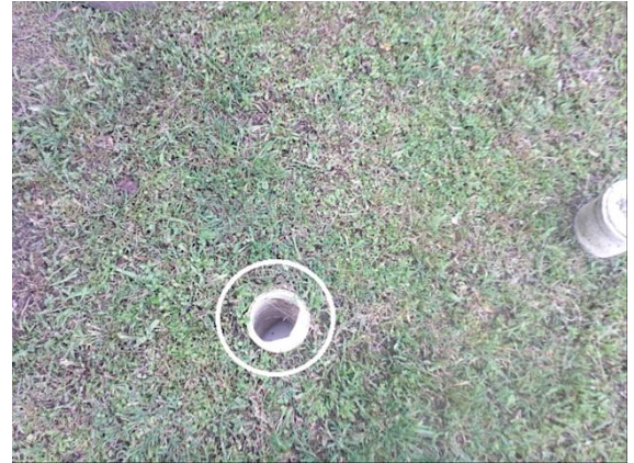
Plumbing: broken cap, replacement or repair
