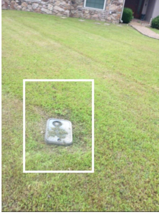
Plumbing: main disconnect
