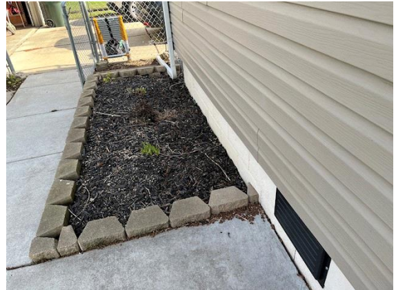
Grading / Drainage: Slight negative slope.
