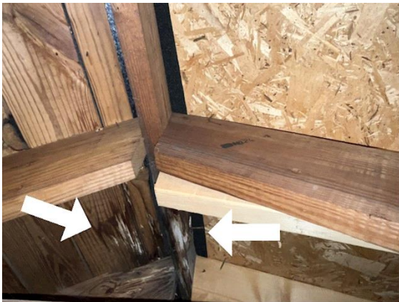
Attic Framing/Sheathing: Possible moisture intrusion.
