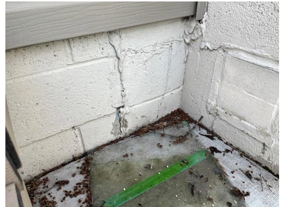
Interior Foundation: Minor crack and deterioration.
