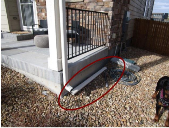
Gutters/Down Spouts: Detached downspout
