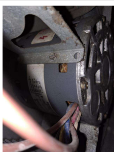
4.3 Item 2 (Picture) Dirty blower
