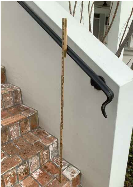
Stairway handrail height is between 34-38"
