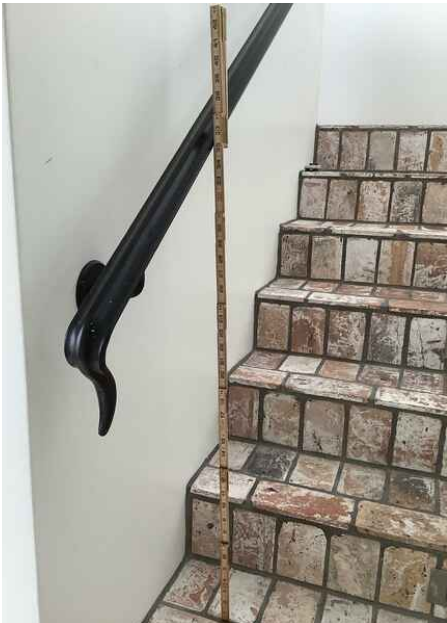
Stairway handrail height is between 34-38"
