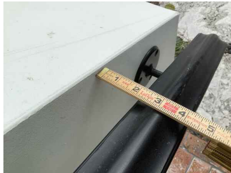
Stairway handrail has at least 1 1/2" min. clear space
