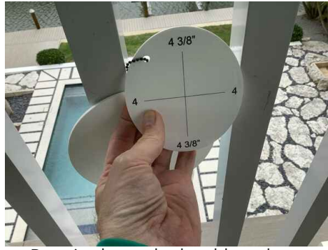
Required guards should not have openings that allow passage of a sphere 4 inches in diameter
