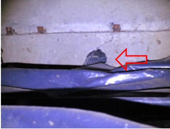
Interior Foundation: hole thru foundation.
