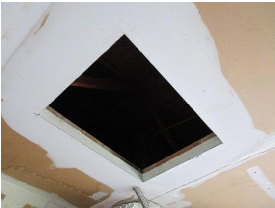
Attic Framing/Sheathing: missing access cover.
