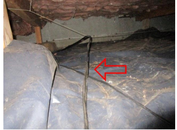
Interior Foundation: electrical wires
