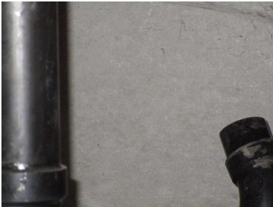
Plumbing: loose pieces of ABS. left over previous work.
