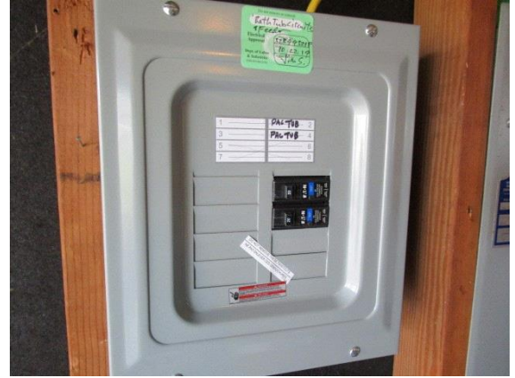
Electrical: Sub panel
