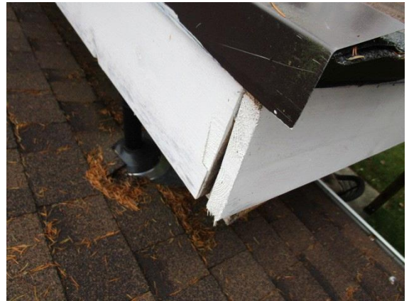
Patio: Patio roof separation in fascia
