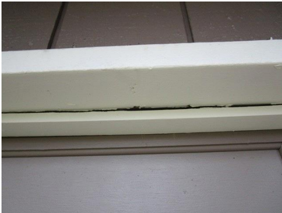
Overhead Garage Doors:
