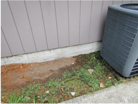
Grading / Drainage: South side negative slope
