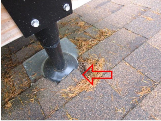
Patio: Patio roof support poorly install under shingles.
