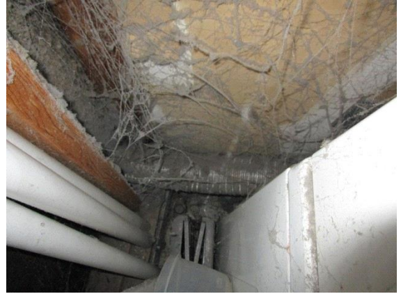
Laundry Facilities: dryer vent.
