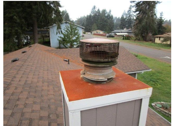
Chimney: Rain cap spark arrester in place at the time of inspection.
