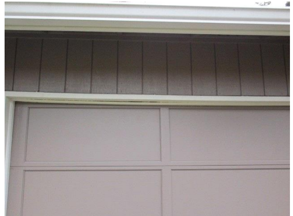
Overhead Garage Doors:
