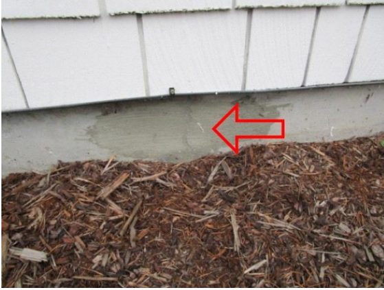
Foundation: crack in foundation.
