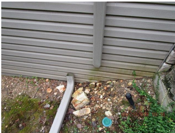
GUTTERS/DOWN SPOUTS: Downspout disconnected
