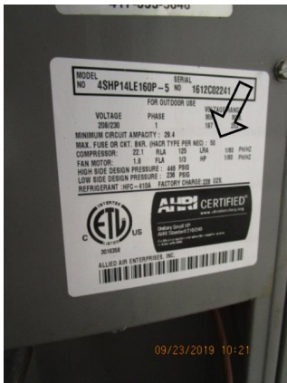
ELECTRICAL: 50 AMP MAX
