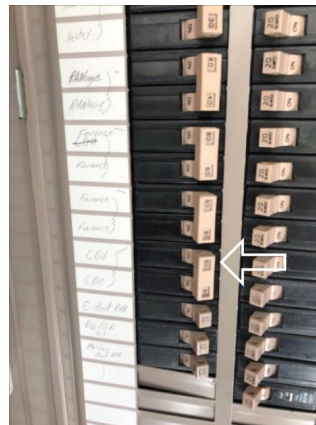
Electrical: 60 AMP Breaker
