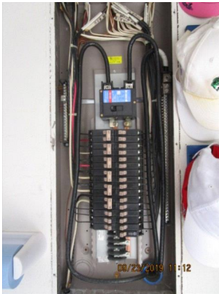
Electrical: Panel with Cover Off
