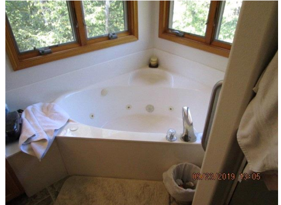
Bathroom: No Access Panel
