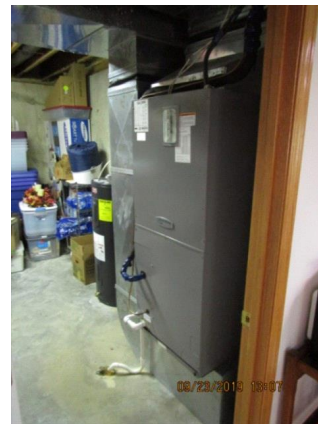
Basement: Furnace, Hot Water & Storage
