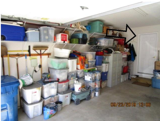
Garage Pedestrian Door into House: No Auto-Closer
