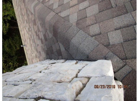
Chimney: Unable to see flashing
