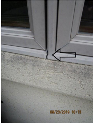
WINDOWS: Cracked Window sill
