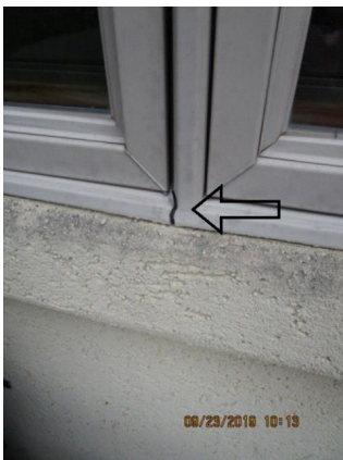
Windows: Cracked Window sill
