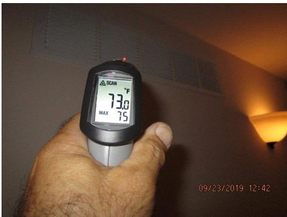
Cooling: Return Air Temp
