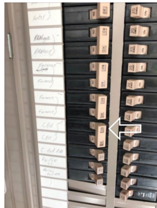
ELECTRICAL: 60 AMP Breaker
