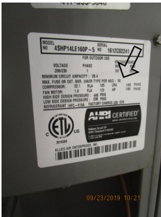
Electrical: 50 AMP MAX
