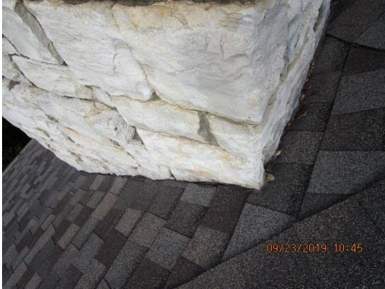
Chimney: Unable to see flashing
