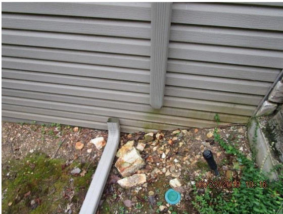
Gutters/Down Spouts: Downspout disconnected
