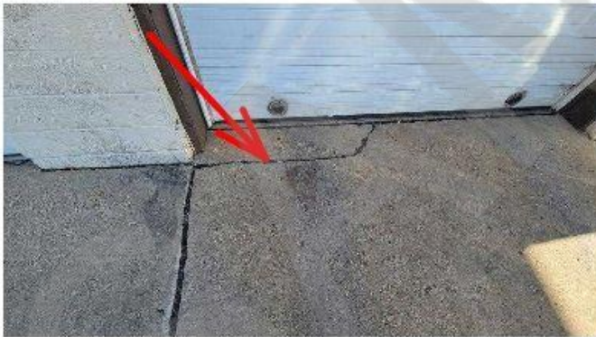
Concrete Parking Lot Crack
