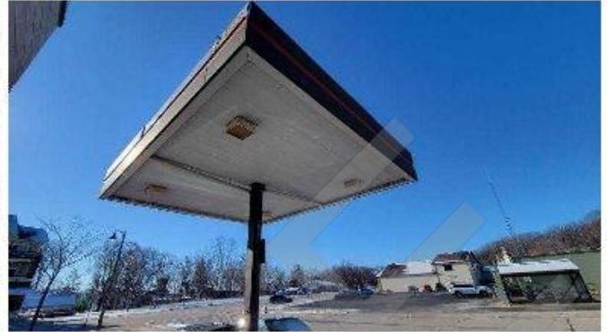
Canopy Lighting Not Inspected
