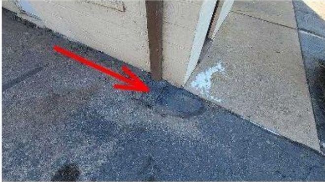
Underground Drain Tile Not Inspected
