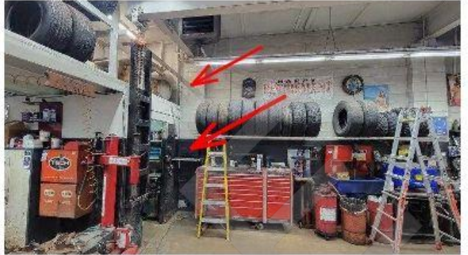
Shop East Wall Previous Water Entry
