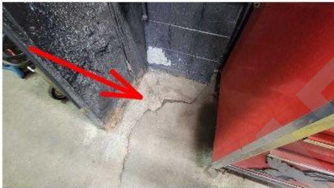
Shop East Ground Previous Water Entry
