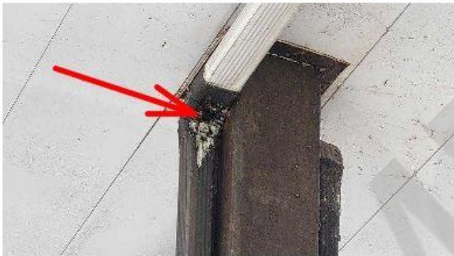
Leaking Canopy Downspout
