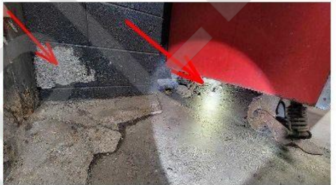
East Shop Wall Deteriorated Block
