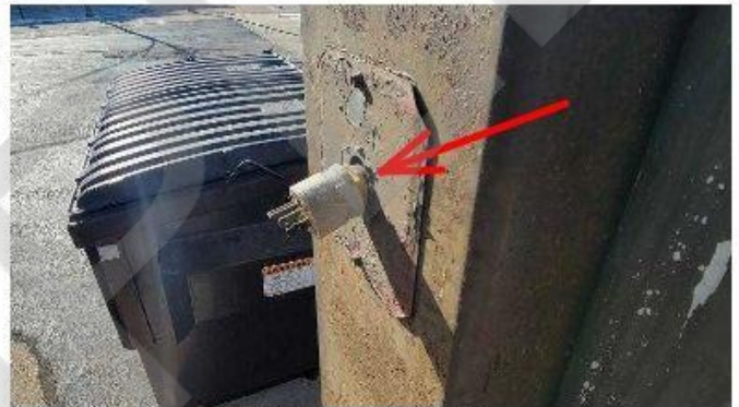
Damaged Canopy Plug
