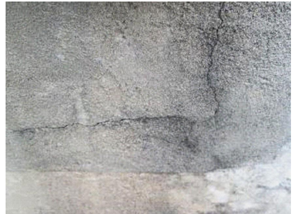
Foundation: Minor cracking.
