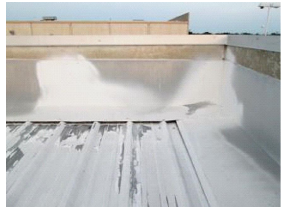
Roofing: High end (east) showing delamination of the elastomeric coating.
