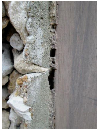
Windows: Gap on window frame stile.
