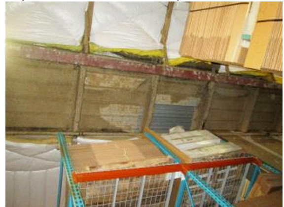
Warehouse Interior: Missing insulation.
