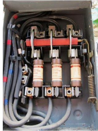
Electrical: Two, 200 amp main service entrance disconnect boxes.
