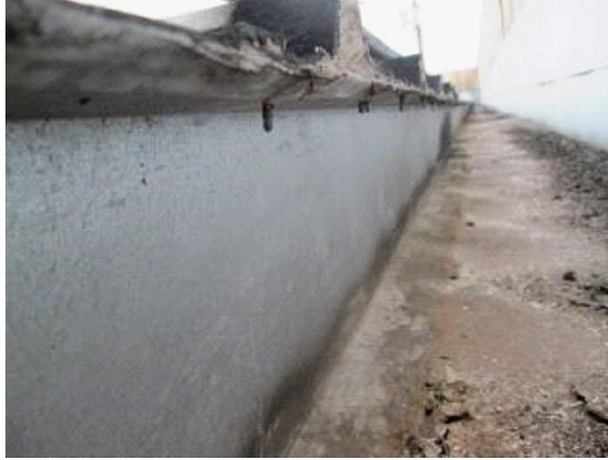
Gutters/Down Spouts: Evidence of water ponding observed on July 22.
