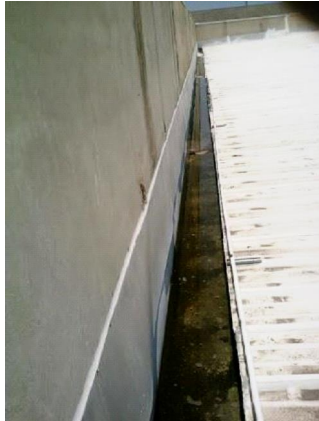
Gutters/Down Spouts: Water ponding observed on July 24, several hours after a light rain.
