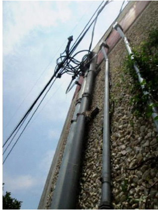
Electrical: Overhead service entrance mast.
