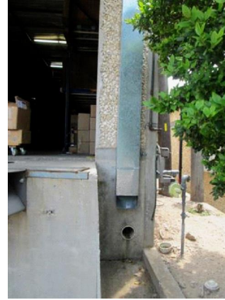
Gutters/Down Spouts: Downspouts and drains on the north and south ends of buildings appear satisfactory.
