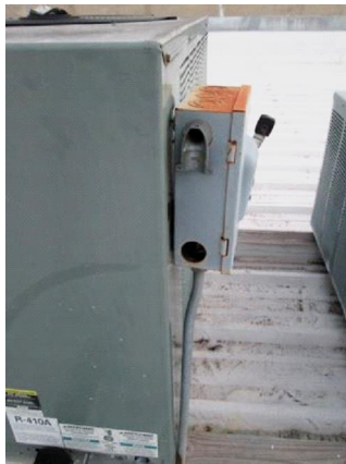
Cooling: Uncovered openings in switch boxes on the 5 ton unit and on one of the 3.5 ton units.
