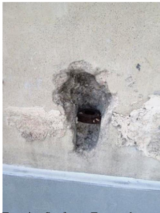
Exterior Surface: Exposed snap tie embedded in concrete inside the west (front) wall above the roof.
