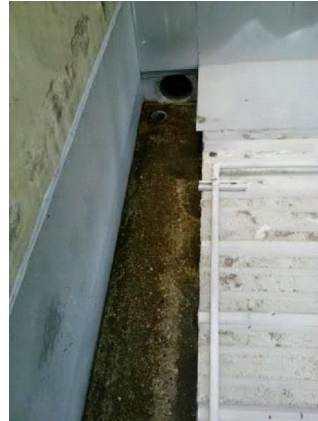
Gutters/Down Spouts: Ponded water near the drains on the north end.
