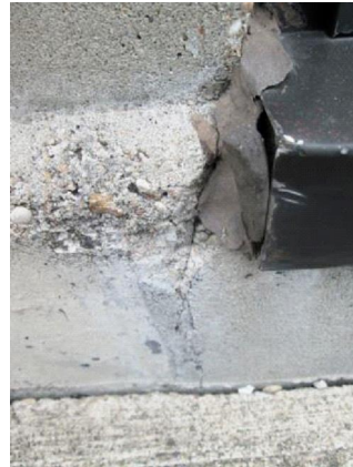
Windows: Open end on window sill.
