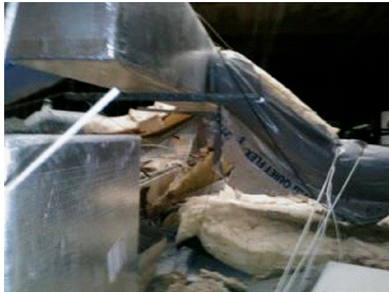
Insulation: Torn insulation on air duct.
