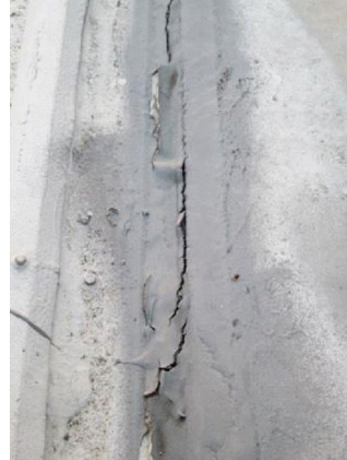
Flashing/Valleys: Cracking of elastomeric coating where flashing meets roof surface.
