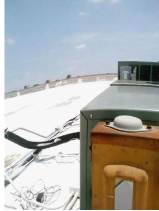
Cooling: Rusted switch box on one of the 3.5 ton units.
