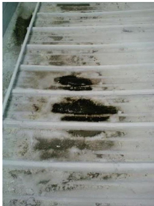
Roofing: Low end (west) where roof meets gutter showing evidence of ponding water.
