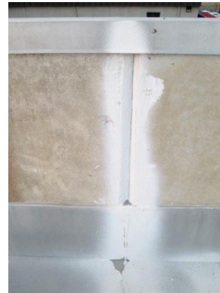
Flashing/Valleys: Coating of seam in side flashing and expansion joint in parapet wall.
