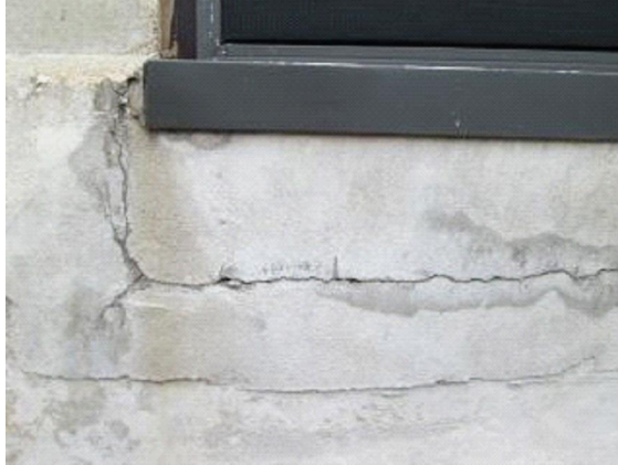
Exterior Surface: Minor crackng under window at west (front) of building.
