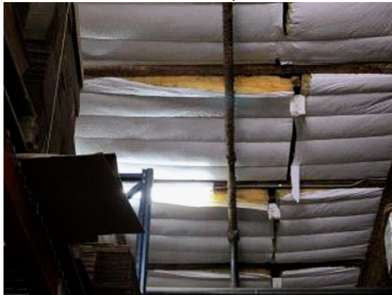
Warehouse Interior: Sagging insulation.
