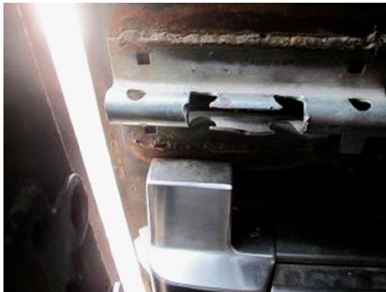
Exterior Doors: Exterior door on back wall at north end does not have functioning hardware. Must be tied after business hours.
