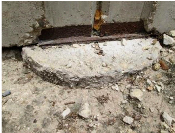
Foundation: Breakage of foundation beam wall over pier.
