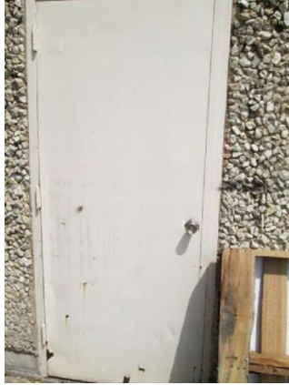
Exterior Doors: Exterior door on front wall at south end next to overhead door. Minor cosmetic damage (typical).
