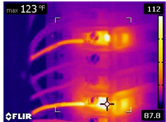
Electrical: Infrared image of electrical panel showing elevated temperatures in the 4th and 7th (from the top) breakers on the left buss bar. Both are 20 amp breakers.
