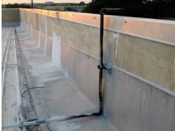
Flashing/Valleys: Cap and side flashing at north parapet wall. Cracking of elastomeric coating where flashing meets roof surface.
