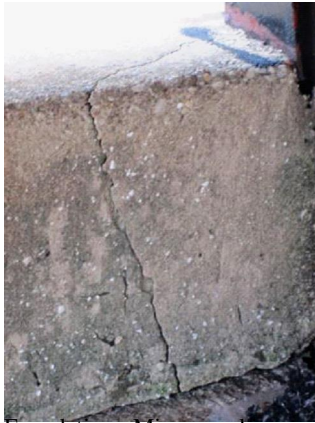
Foundation: Minor cracking.
