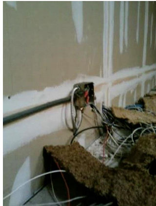
Attic Electrical: Open junction box above ceiling grid.
