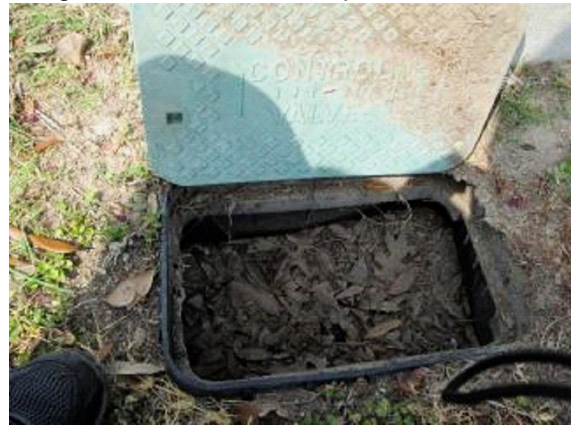
Plumbing: Dirt covering shut-off.
