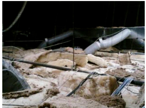
Attic Electrical: Wires on insulation above ceiling grid.
