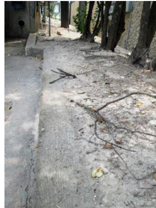
Grading / Drainage: Positive slope on south (right) wall.
