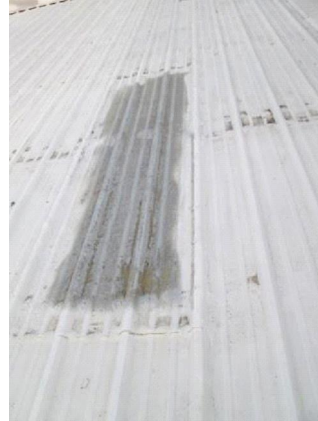
Roofing: Translucent panel cut into roof. Possible safety hazard.
