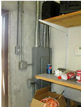
Electrical: Main panel obstructed by adjustable shelving.
