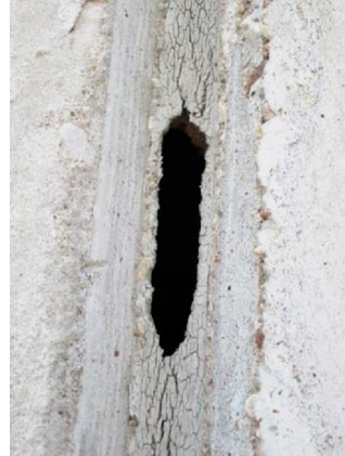
Exterior Surface: Gap and cracking of sealant in expansion joint between wall sections.
