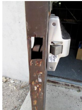
Exterior Doors: Another view of exterior door on back wall at north end.
