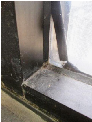
Windows: Loose gasket in window.
