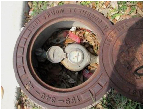
Plumbing: Water meter.
