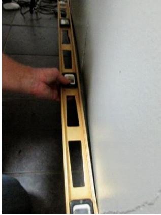
Interior Rooms (showroom, offices, conference room, and restroom.: Level used as straight edge to illustrate bow in wall.
