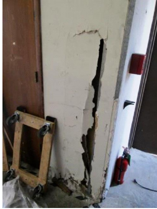
Warehouse Interior: Sheetrock damage.
