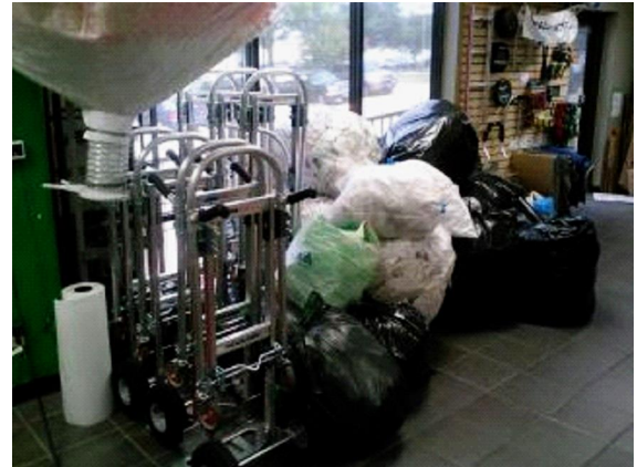
Heating: Obstructions preventing inspection of furnace.
