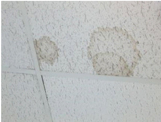
Interior Rooms (showroom, offices, conference room, and restroom.: Typical ceiling stains.
