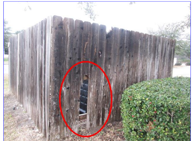
2.8 Item 2 damaged pickets
