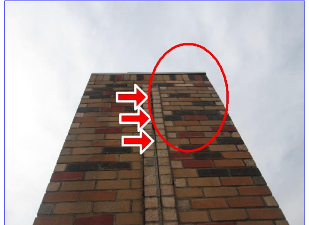
E. Item 2 chimney brick repair needed
