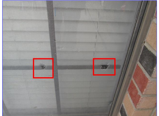
I. Item 9 damaged screens
