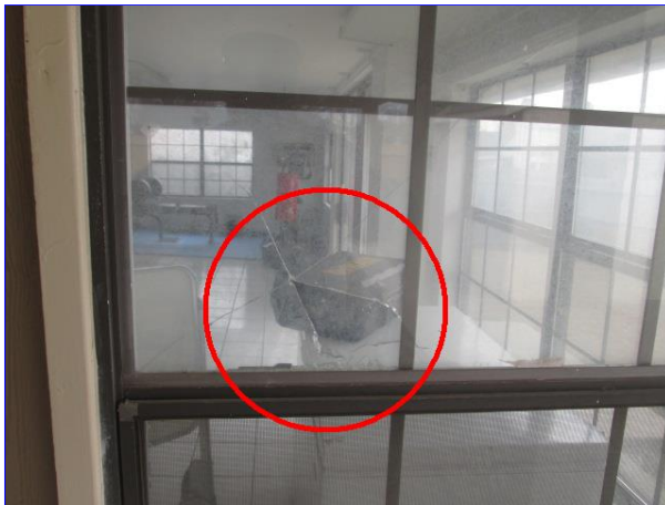
I. Item 11 broken glass, patio
