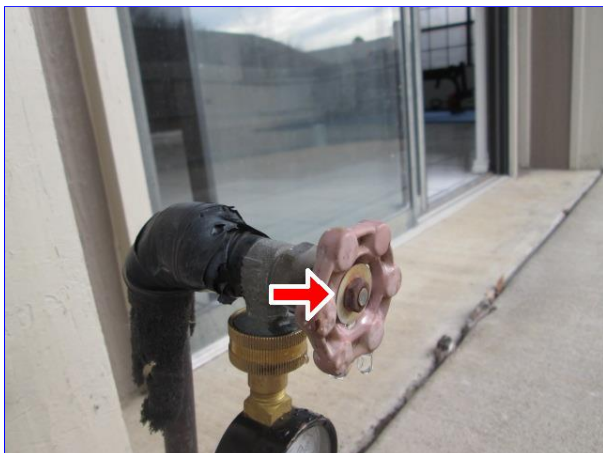
A. Item 7 leaking at handle
