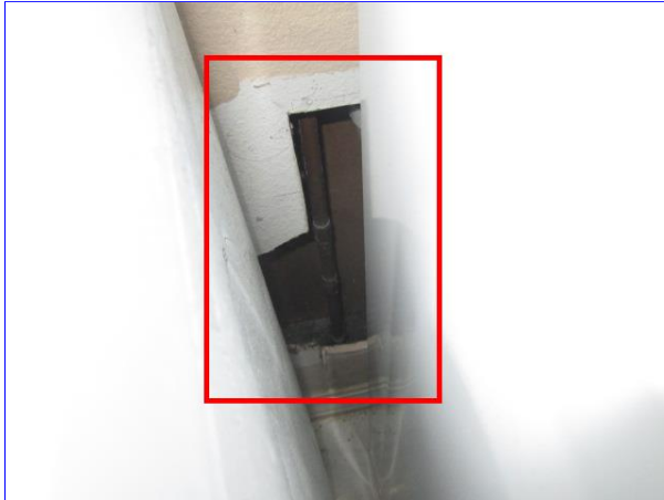
E. Item 15 large hole in wall.
