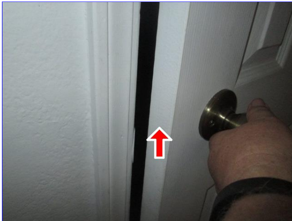
G. Item 8 no latch at bedroom closet
