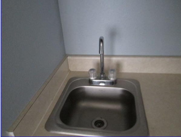
A. Item 3 faucet not operating
