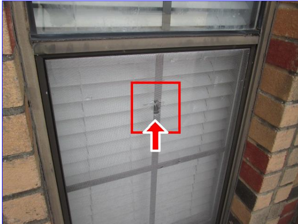
I. Item 8 damaged screens
