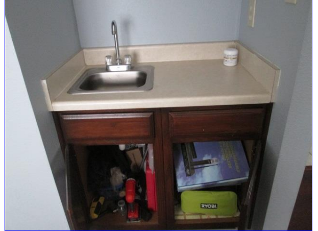
A. Item 4 faucet not operating
