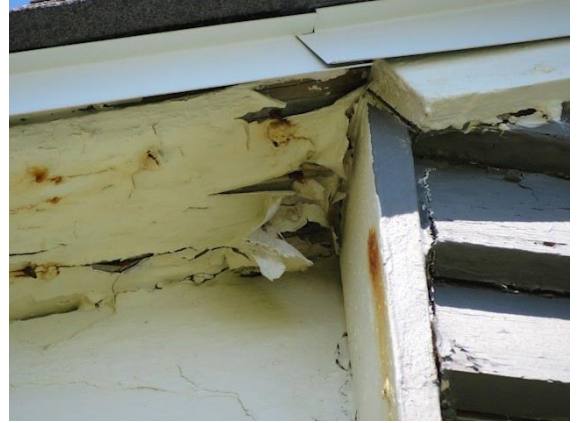
Exterior Surface: View of water damaged eaves around home
