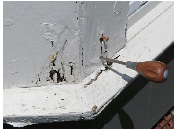
Windows: Views of damaged wooden window frames
