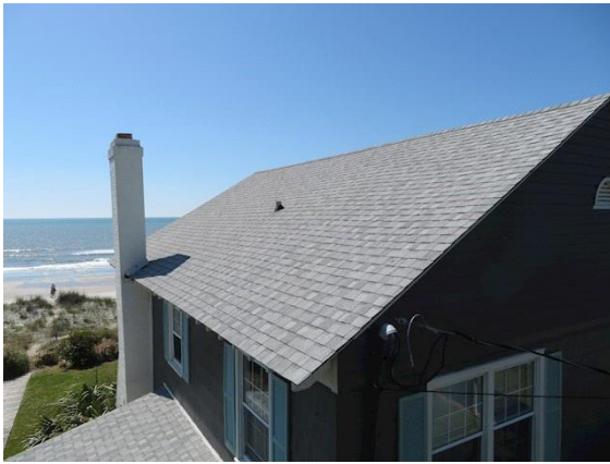
Chimney: View of left chimney pulling away from house
