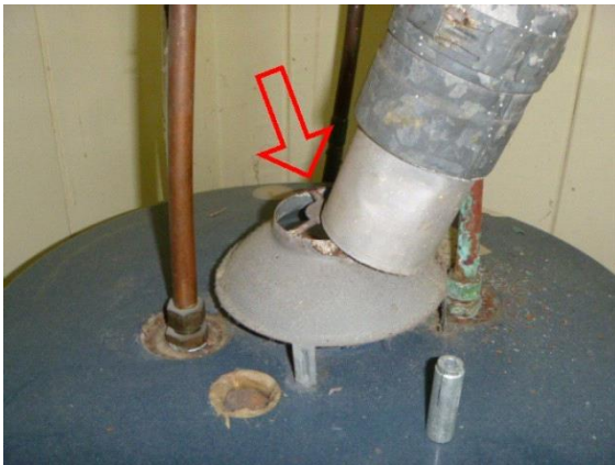
Water Heater: View of flue not properly aligned on top of water heater
