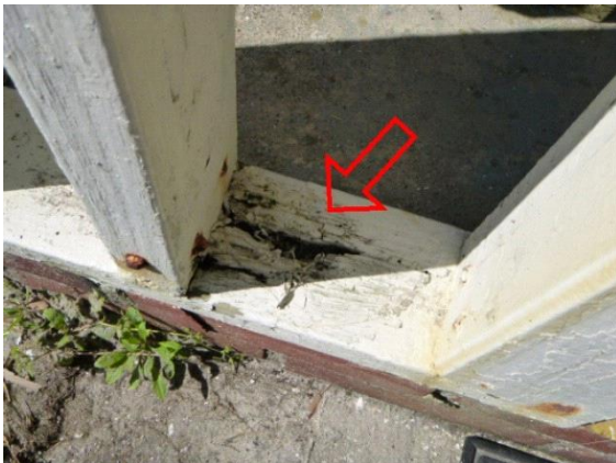
Left Covered Porch: View of soft water damaged wood on base of guardrails
