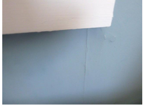
Upstairs Rear Right Bedroom: View of settlement cracks in walls above and below windows
