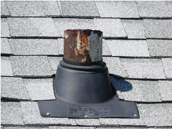
Flashing/Valleys: Views of heavily corroded plumbing vents and flashing with exposed nail heads
