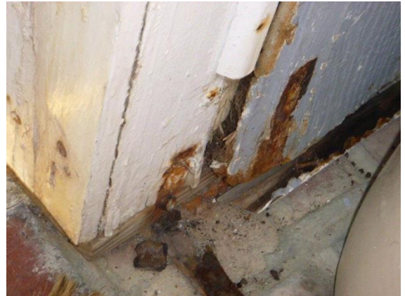
Exterior Doors: View of water damaged wood on base of rear door frame
