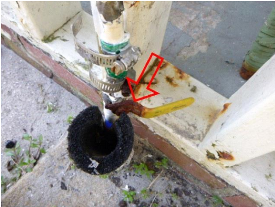
Exterior Surface: View of rusted water valve on exterior water faucet
