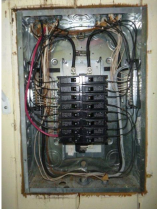
Electrical: View of electric sub panel located in the laundry room
