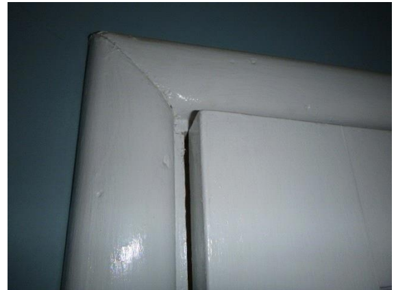
Upstairs Front Right Bedroom: View of bedroom entry door hitting top of door frame
