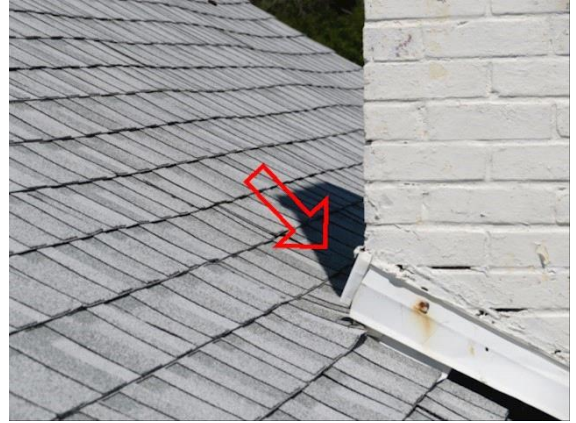
Chimney: View showing where a roof cricket needs to be installed when a chimney is wider than 30 inches wide
