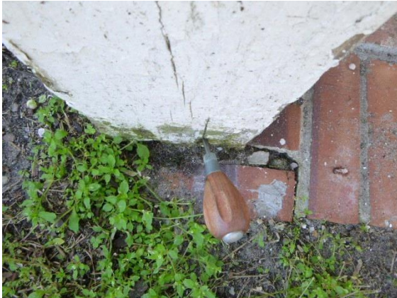
Front Brick Patio: Views of water damaged wood at base of columns
