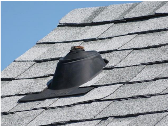
Flashing/Valleys: Views of heavily corroded plumbing vents
