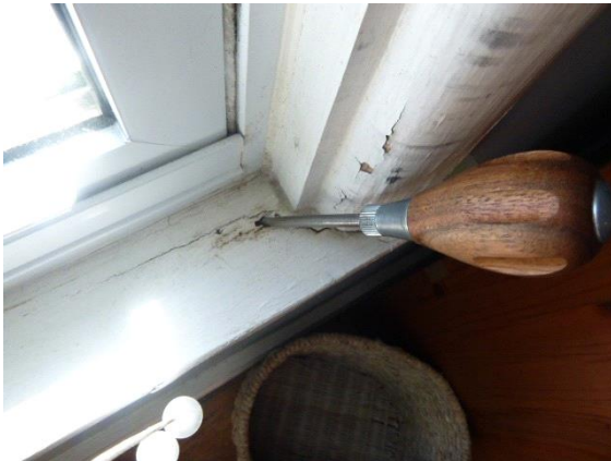
Upstairs Front Right Bedroom: View of water damaged window sill
