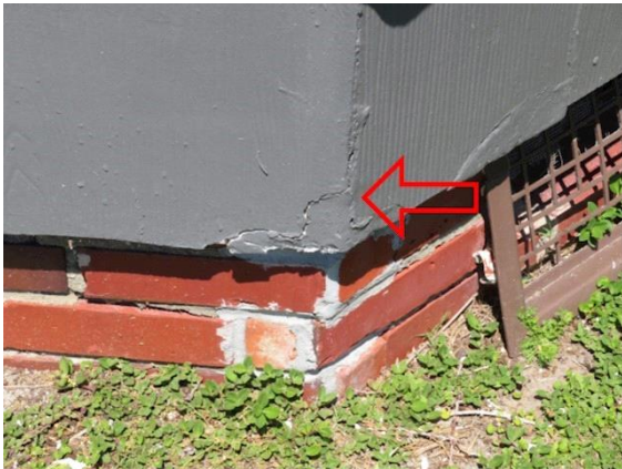
Exterior Surface: Views of cracked composite siding
