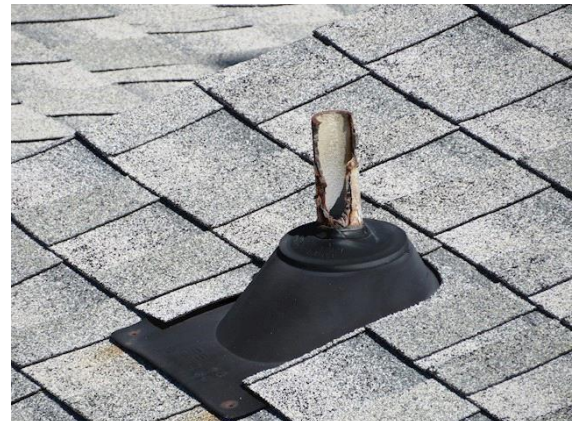
Flashing/Valleys: Views of heavily corroded plumbing vents and flashing with exposed nail heads
