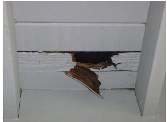
Right Enclosed Porch: Views of soft, water damaged wood present on walls and ceiling of enclosed porch
