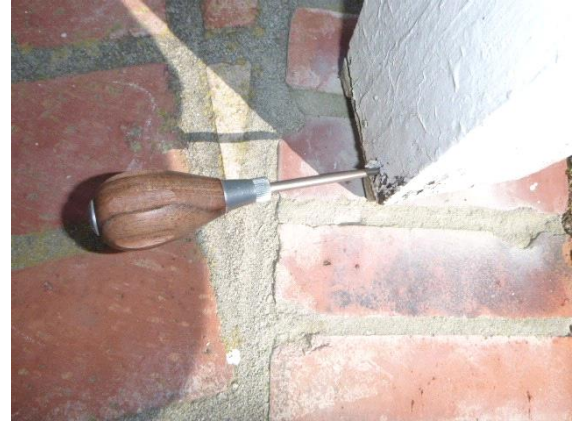
Front Brick Walkway: View of soft water damaged wood at base of support post
