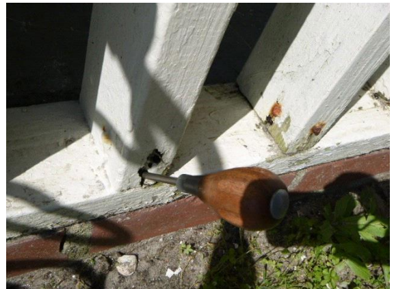
Left Covered Porch: View of soft water damaged wood on base of guardrails
