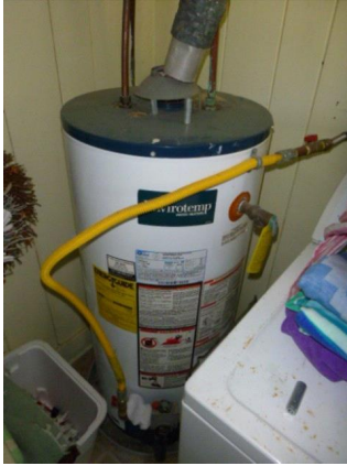
Water Heater: Overall view of water heater located in laundry room
