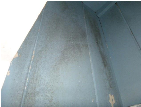
Upstairs Hall Closet: Views of microbial growth in upstairs hall closet
