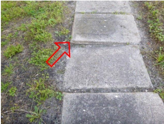
Paver Walkway: View showing height differential of paver walkway
