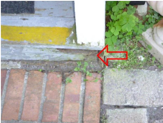
Front Stoop: Views of water damaged wood trim
