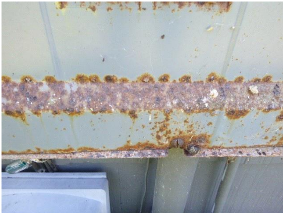
Electrical: View of excessive corrosion on main electrical panel
