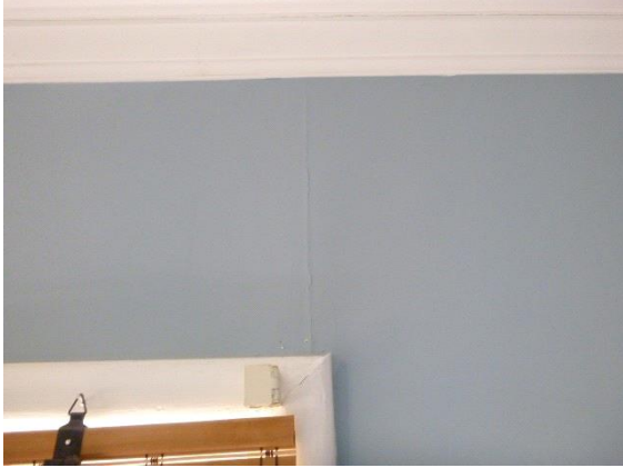
Upstairs Rear Right Bedroom: View of settlement cracks in walls above and below windows
