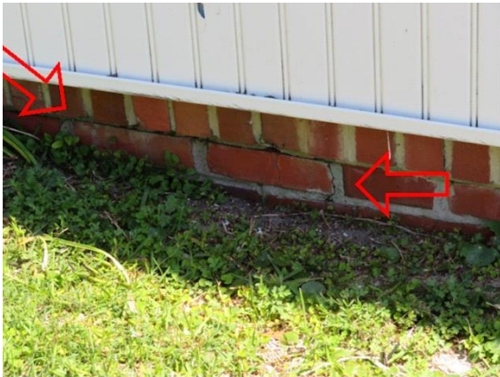
Foundation - Slab: Views of cracks in mortar on brick foundation wall
