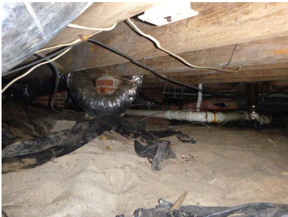
Interior Foundation: Views showing ductwork, plumbing and ground to joist clearance in crawl space
