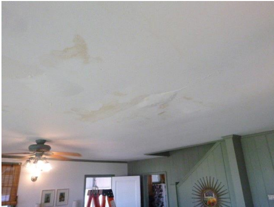
Living Room: Overall view of water stain on living room ceiling
