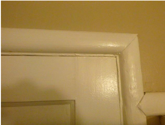
Downstairs Bathroom: View of bathroom entry door sticking in door frame
