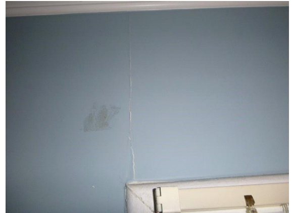
Upstairs Front Left Bedroom: View of settlement cracks in walls above and below windows
