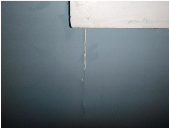
Upstairs Front Left Bedroom: View of settlement cracks in walls above and below windows
