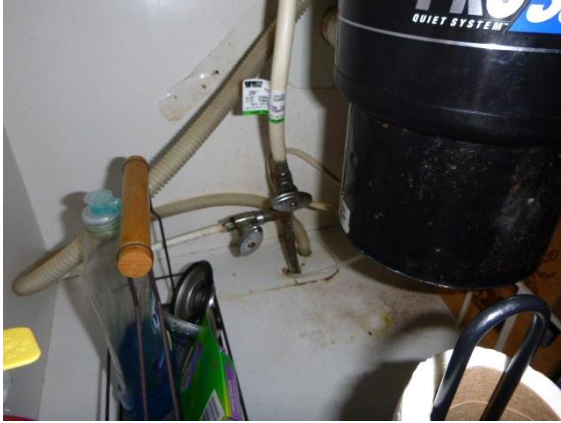
Plumbing: Overall view of plumbing pipes below sinks
