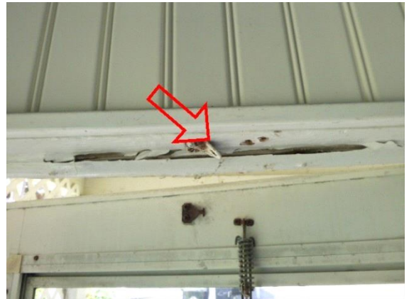
Exterior Doors: View of damaged wood trim on front storm door frame
