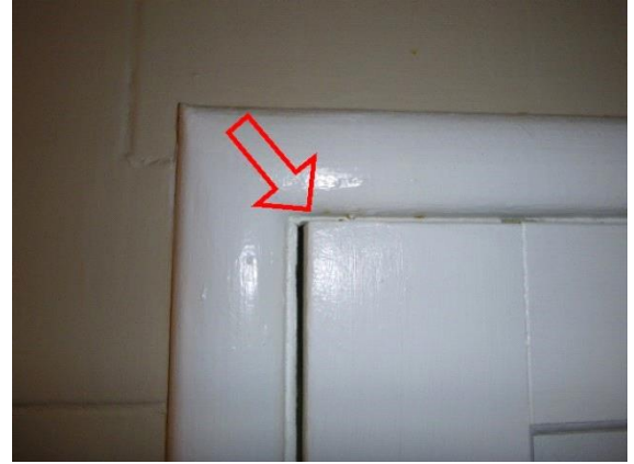
Exterior Doors: View of wooden side entry door hitting top of door frame when closing
