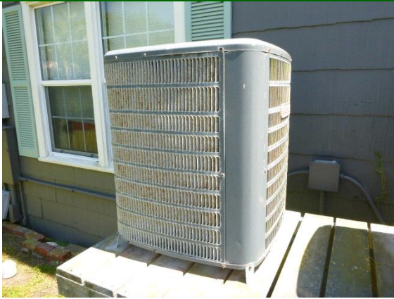
Upstairs Cooling: View of HVAC condenser located on the front side of the house
