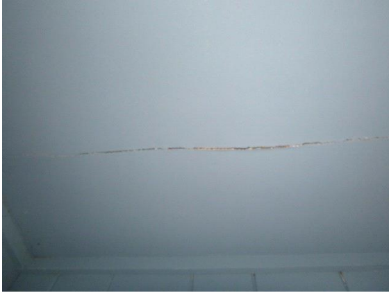
Upstairs Front Right Bedroom: View of cracked ceiling in bedroom closet
