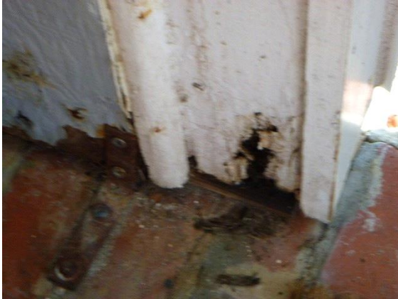
Exterior Doors: View of water damaged wood on base of rear door frame
