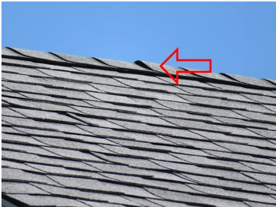
Roofing: View of lifted asphalt roof shingles due to roofing nails lifting out of sheathing
