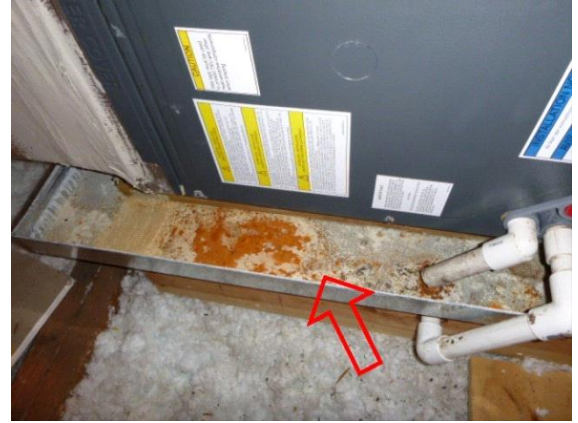
Upstairs Cooling: View of corrosion in catch pan under air handler located in attic
