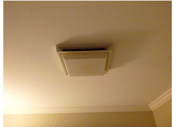
Downstairs Bathroom: View of defective bathroom exhaust fan and ceiling light
