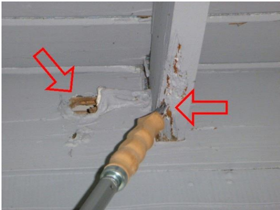
Right Enclosed Porch: Views of soft, water damaged wood present on walls and ceiling of enclosed porch
