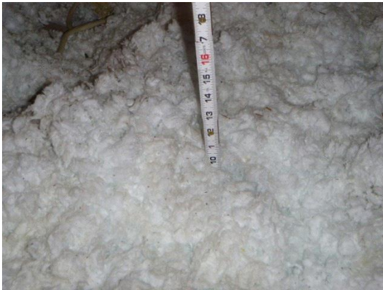
Attic Insulation: View showing the depth of insulation located in the attic
