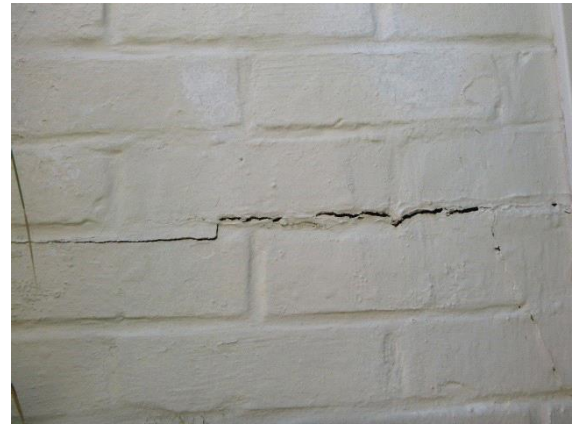
Chimney: View of cracked mortar on left chimney
