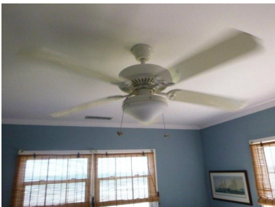
Upstairs Rear Right Bedroom: View of defective fan light in bedroom
