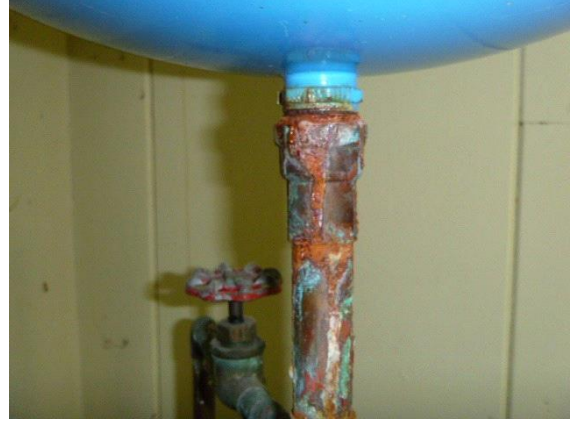
Water Heater: View of excessive corrosion present at base of the fitting located at the top of water heater
