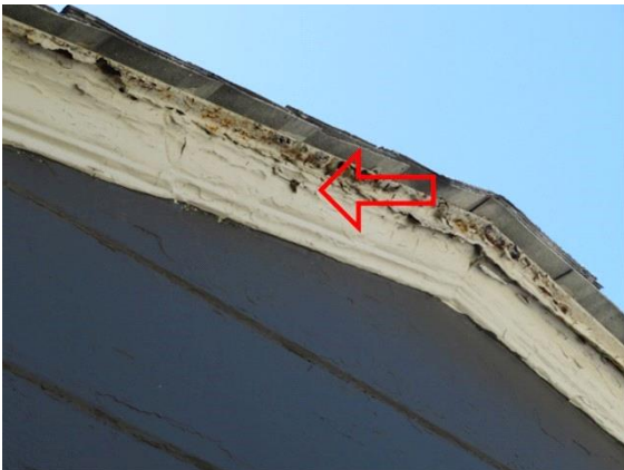
Exterior Surface: View of water damaged rake board on front of home
