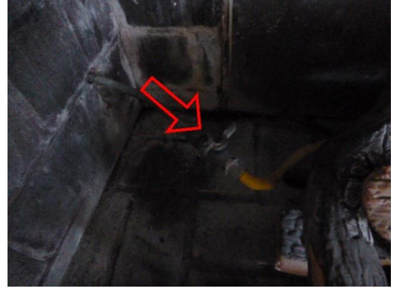
Fireplace/Stove: View showing the gas valve located inside the fireplace that is in the off position
