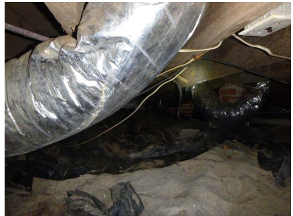
Interior Foundation: Views showing ductwork, plumbing and ground to joist clearance in crawl space
