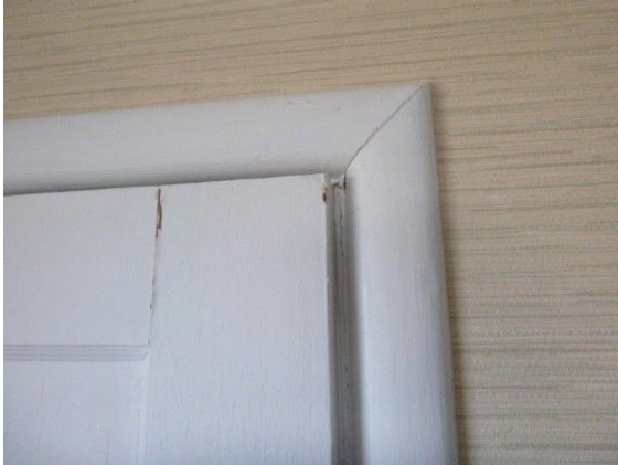
Upstairs Right Bathroom: View of bathroom entry door hitting top of door frame
