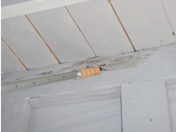
Right Enclosed Porch: Views of soft, water damaged wood present on walls and ceiling of enclosed porch
