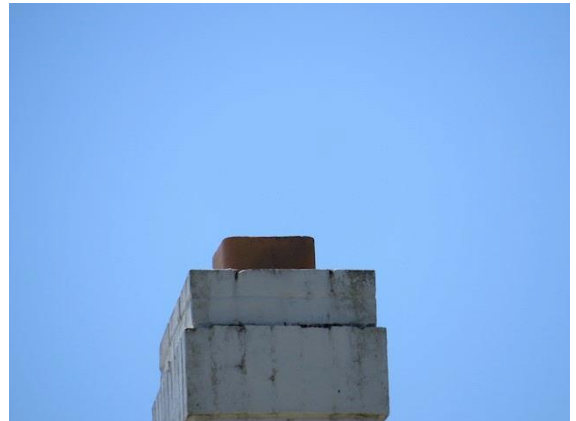
Chimney: View of missing rain cap
