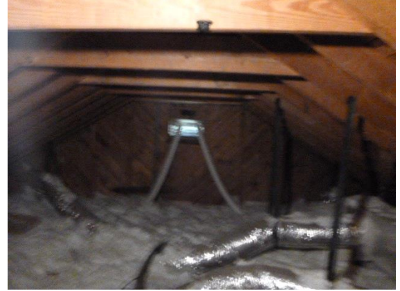
Attic Ventilation: View of gable vents located on each end of attic
