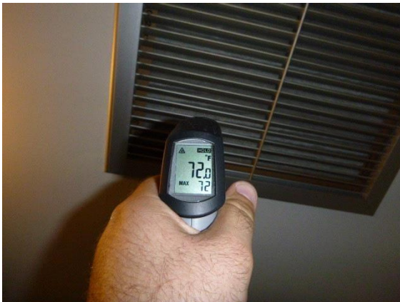
Upstairs Cooling: View of return air temperature using a digital thermometer in the cooling mode
