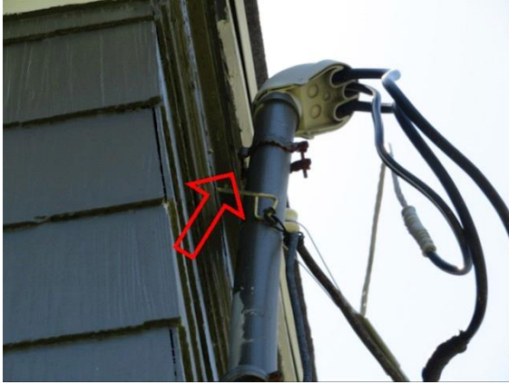
Electrical: Views of detached/corroded brackets on electrical mast
