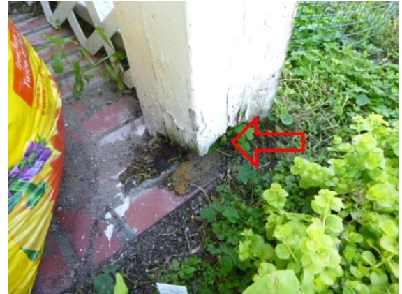
Front Brick Patio: Views of water damaged wood at base of columns
