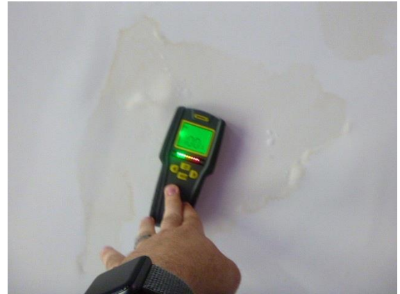
Living Room: Overall view of water stain on living room ceiling with moisture meter
