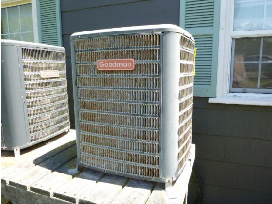
Downstairs Cooling : View of HVAC condenser located on the front side of the house
