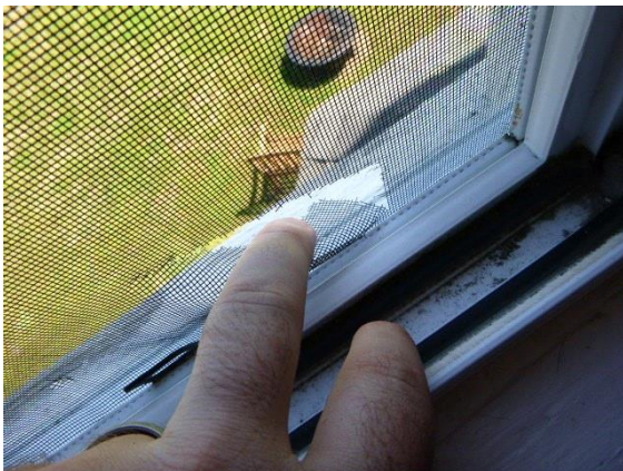
Upstairs Rear Left Bedroom: View of hole in bedroom window screen
