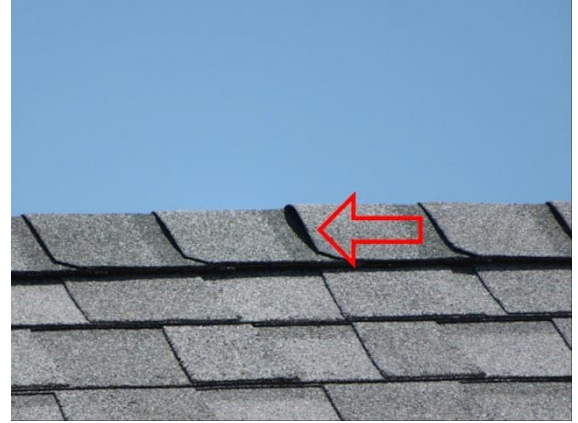
Roofing: View of lifted asphalt roof shingles due to roofing nails lifting out of sheathing
