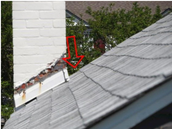
Chimney: View showing where a roof cricket needs to be installed when a chimney is wider than 30 inches wide
