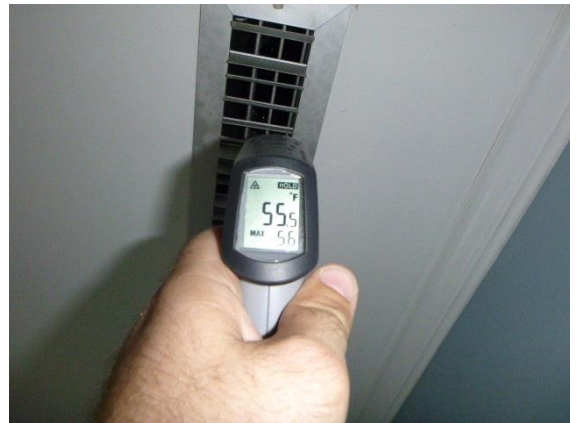
Upstairs Cooling: View of supply air temperature using a digital thermometer in the cooling mode
