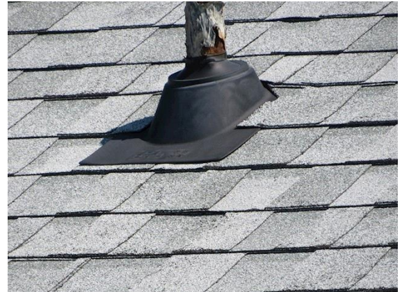
Flashing/Valleys: Views of heavily corroded plumbing vents
