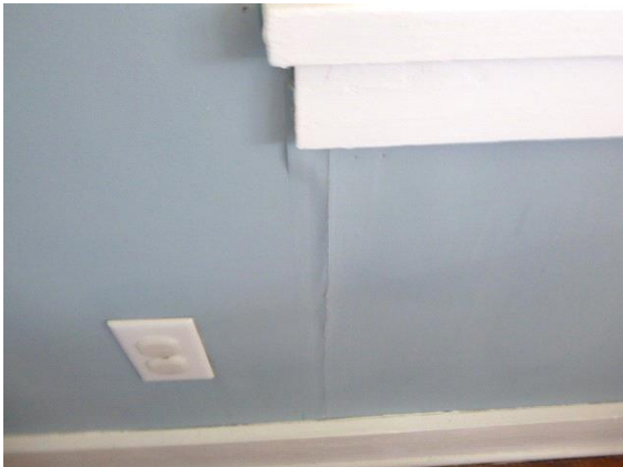
Upstairs Rear Right Bedroom: View of settlement cracks in walls above and below windows
