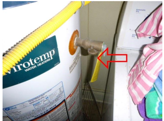
Water Heater: View of missing TPR valve extension pipe on the side of water heater
