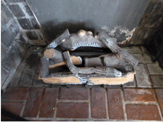
Fireplace/Stove: Overall view of gas log fireplace in living room
