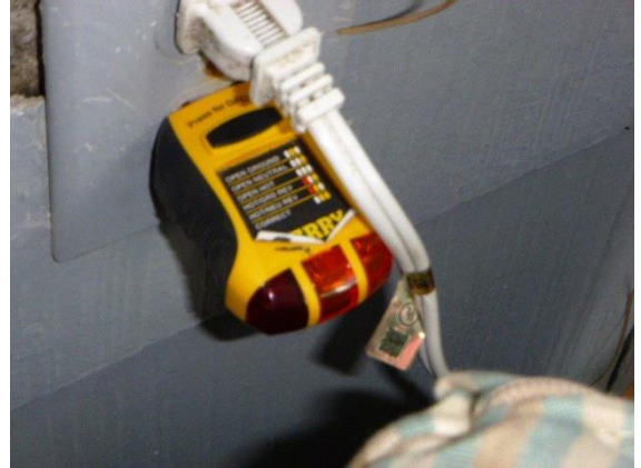
Right Enclosed Porch: View of wall receptacle with no power
