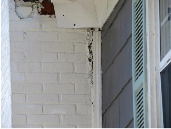
Chimney: View of left chimney pulling away from exterior wall
