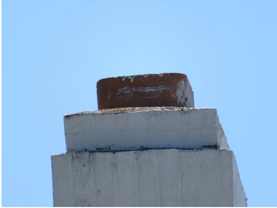
Chimney: View of missing rain cap
