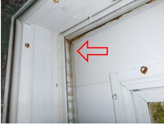
Exterior Doors: View of side entry storm door hitting frame when closing
