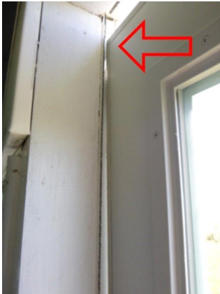
Exterior Doors: View of rear storm door hitting frame when closing
