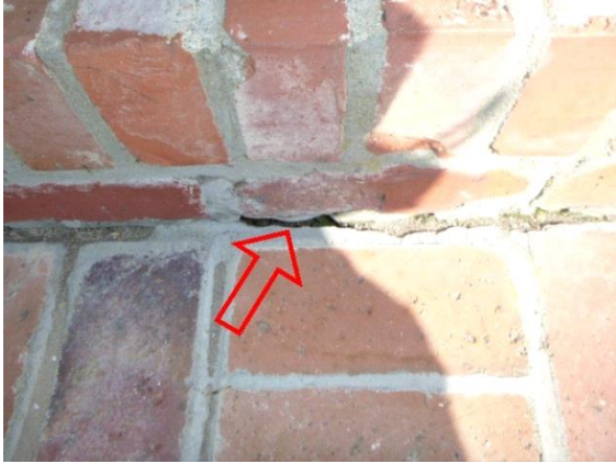
Front Brick Walkway: View of cracked mortar on front brick walkway
