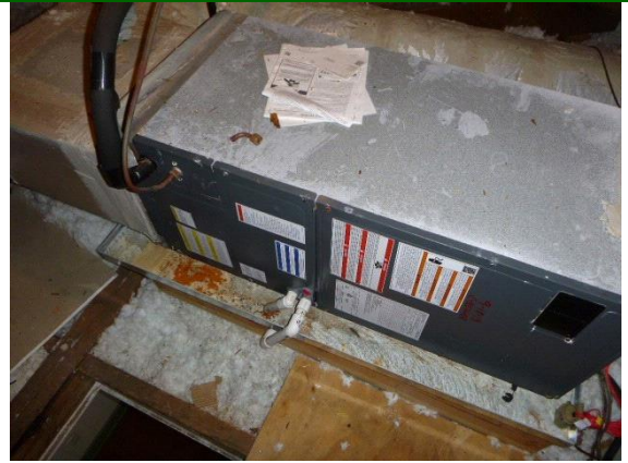
Upstairs Cooling: View of air handler located in the attic area
