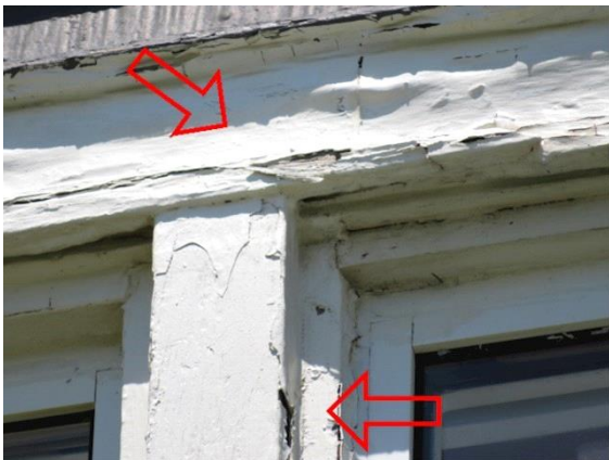
Windows: Views of damaged wooden window frames
