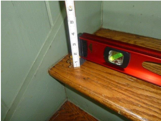
Stairs / Railings: View showing negative pitch on stairs
