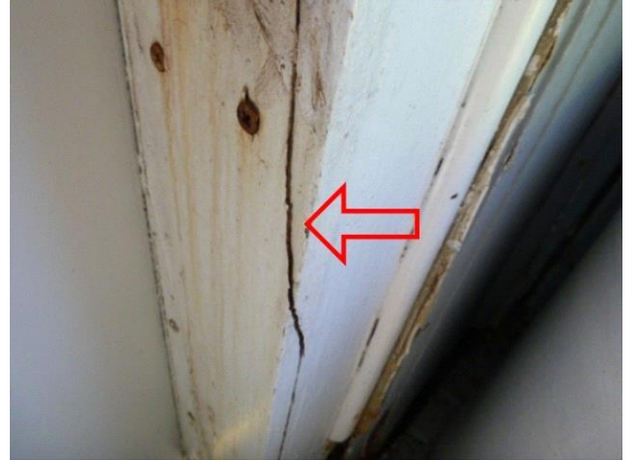
Exterior Doors: View of cracked rear door frame
