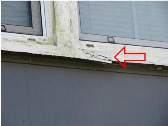
Windows: Views of damaged wooden window frames
