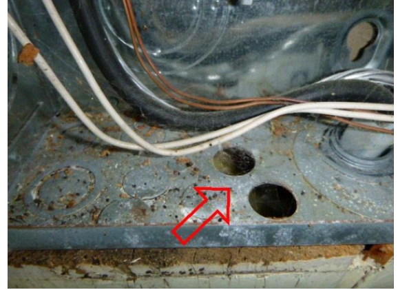
Electrical: View of open knock outs located at the bottom of the electric sub panel
