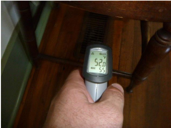
Downstairs Cooling : View of supply air temperature using a digital thermometer in the cooling mode
