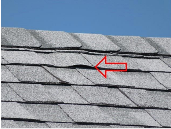
Roofing: View of lifted asphalt roof shingles due to roofing nails lifting out of sheathing
