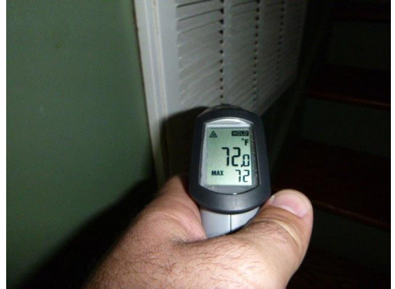
Downstairs Cooling : View of return air temperature using a digital thermometer in the cooling mode
