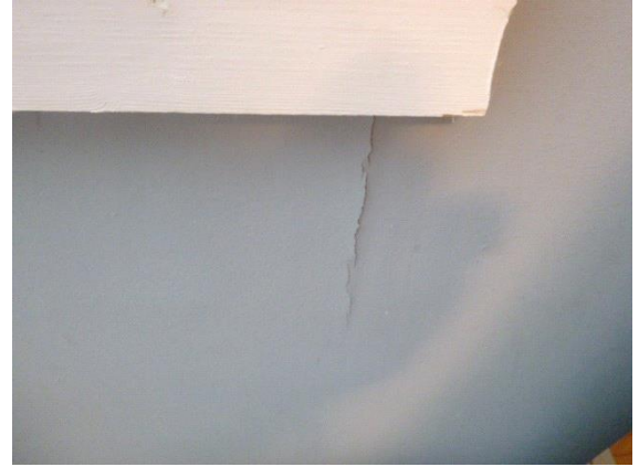
Upstairs Front Right Bedroom: View of wall crack below bedroom window
