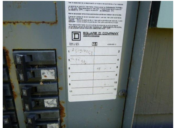
Electrical: View of main panel not labeled
