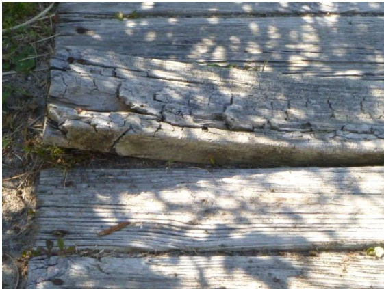
Rear Wood Walkway: View of bowed tread board on rear wood walkway
