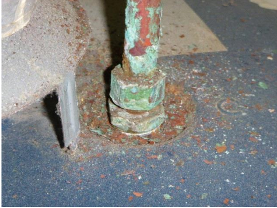
Water Heater: View of excessive corrosion present at base of the fitting located at the top of water heater
