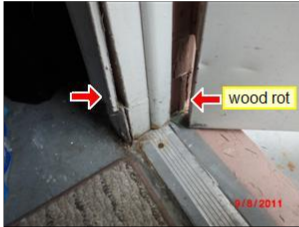
3.3 Picture 1 rotted door frame
