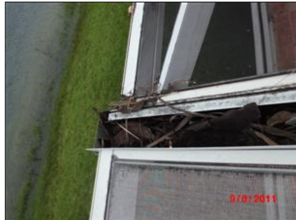
2.4 Picture 2 clogged gutter
