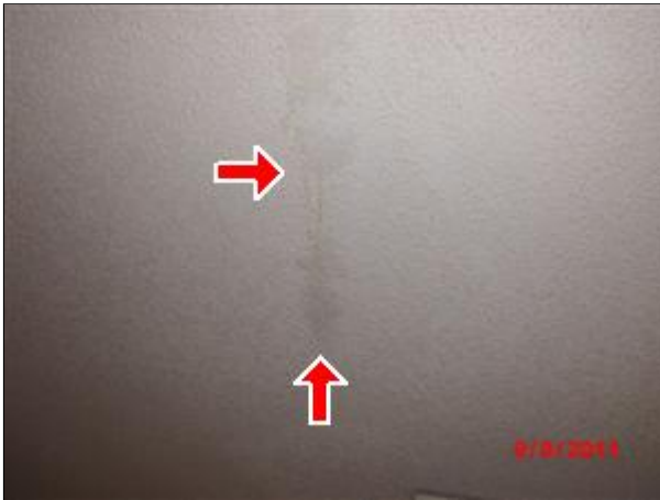
12.0 Picture 1 a/c leak from attic
