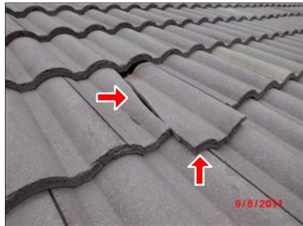
2.0 Picture 2 broken tiles
