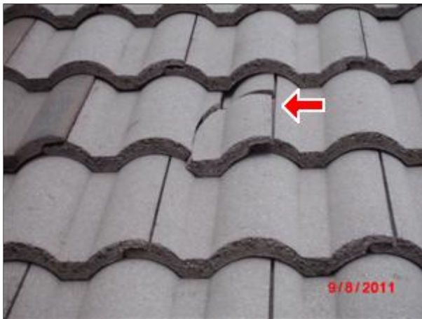
2.0 Picture 1 broken tiles front
