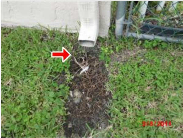
2.4 Picture 1 missing splash stone
