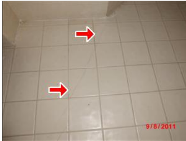
10.2 Picture 1 crack tiles
