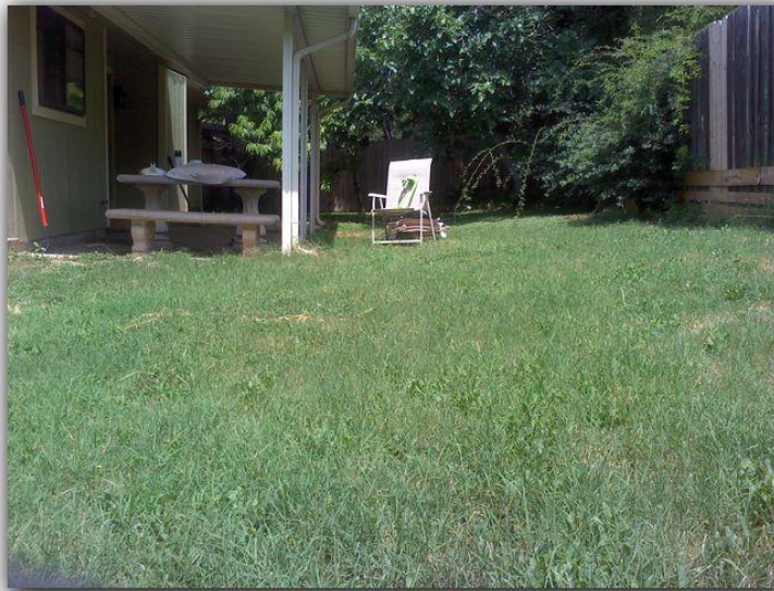
Backyard slope toward foundation.
