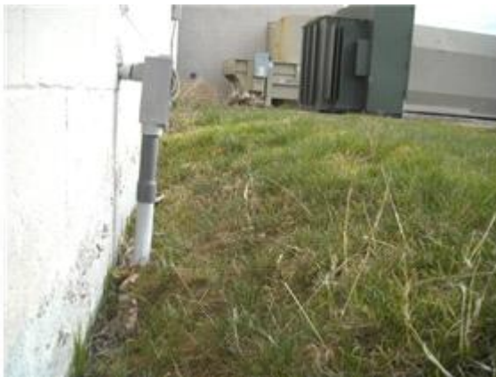
Foundation: Damage to the base of the marquis
