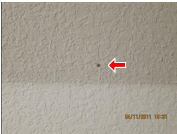
F. Picture 1 Nail pop in ceiling master bedroom
