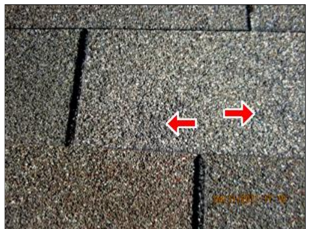
C. Picture 4 Light hail damage
