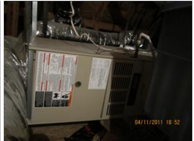
A. Picture 2 Heating equipment
