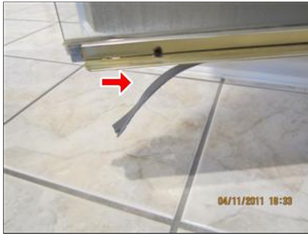
G. Picture 3 Rubber gasket torn on master shower door
