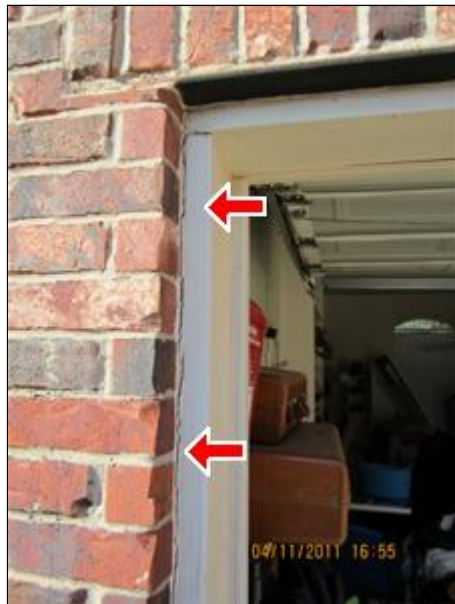
G. Picture 1 Sealant separation
