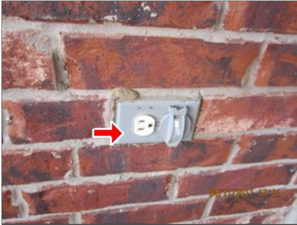
B. Picture 1 Exterior outlet missing cover
