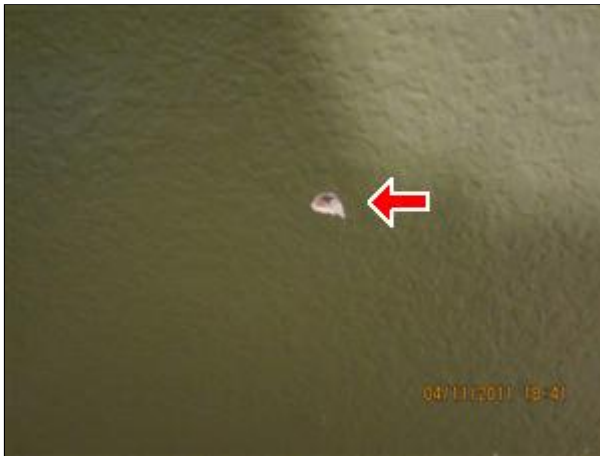
E. Picture 15 Hole in wall
