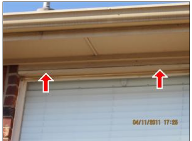
H. Picture 2 Sealant separation
