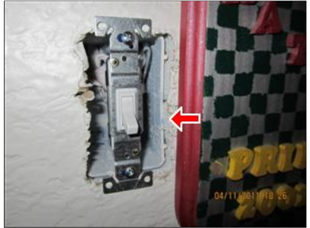
B. Picture 2 Switch cover plate missing
