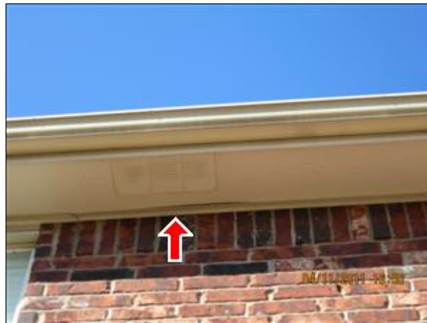
E. Picture 1 Sealant separation
