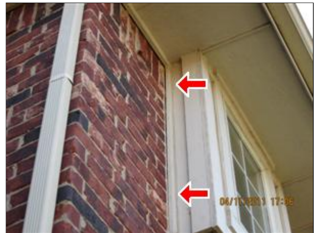
E. Picture 6 Sealant separation
