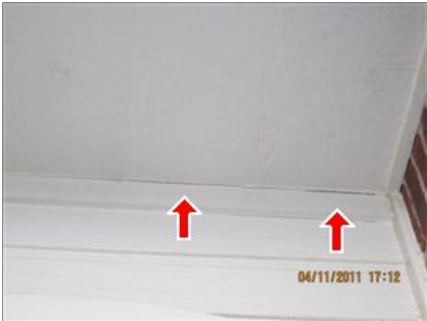
E. Picture 8 Sealant separation
