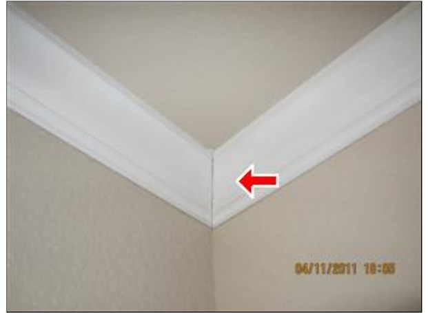
E. Picture 14 Sealant separation at corner joints in crown mold
