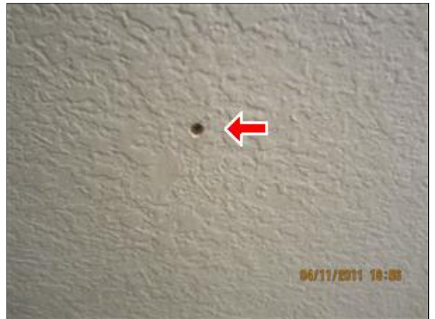
E. Picture 16 Nail pop at stair well
