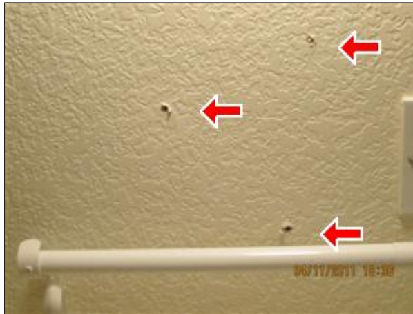
F. Picture 3 Nail pops in master closet
