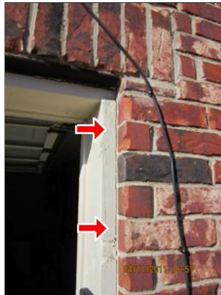
G. Picture 2 Sealant separation
