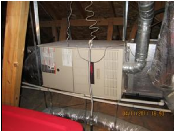
A. Picture 1 Heating equipment
