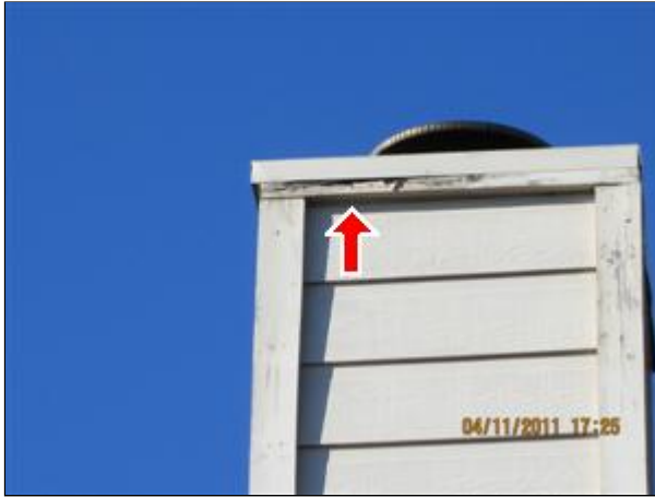
J. Picture 1 Paint peeling on wood trim
