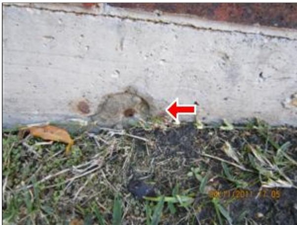
A. Picture 3 Cable end exposed
