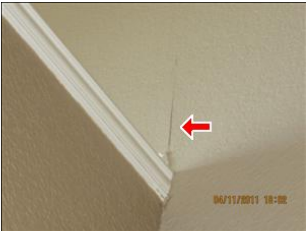
E. Picture 11 Crack in wall above front entry
