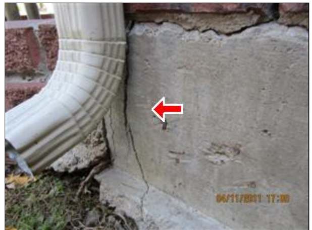
A. Picture 4 Corner crack
