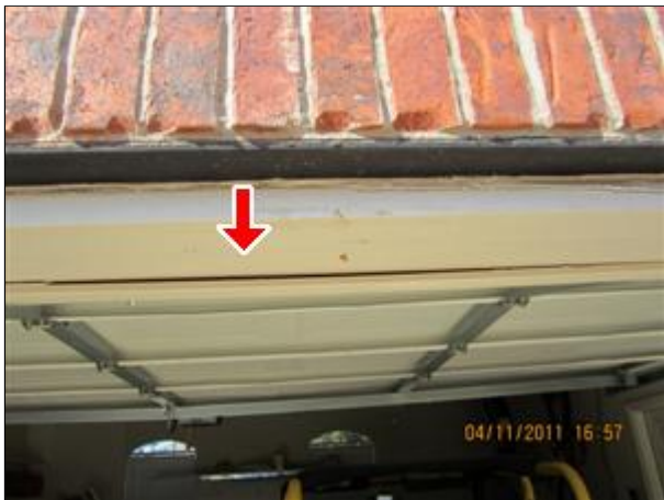
E. Picture 9 Wood trim coming loose
