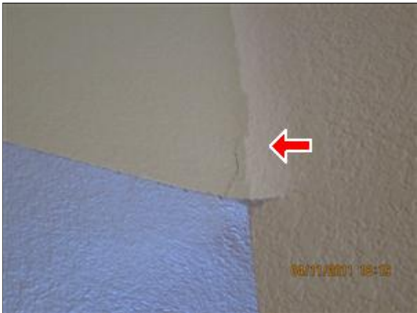
E. Picture 12 Crack in wall at kitchen/living room
