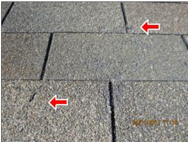
C. Picture 1 Light hail damage
