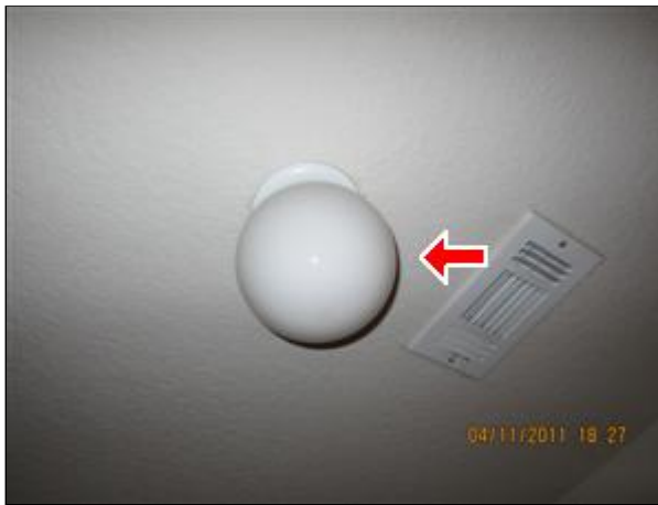
B. Picture 3 Fixture not working
