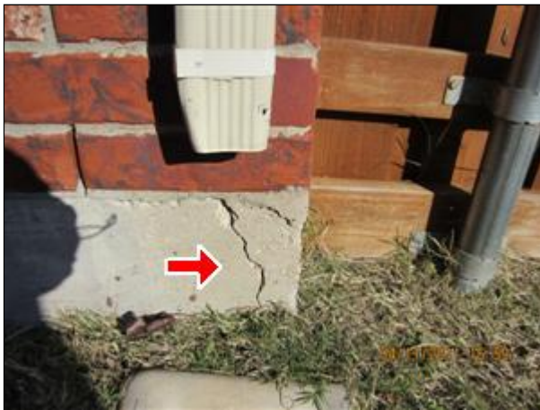
A. Picture 1 Corner Crack
