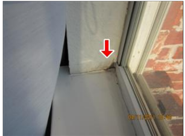
H. Picture 4 Moisture damage to inside window
