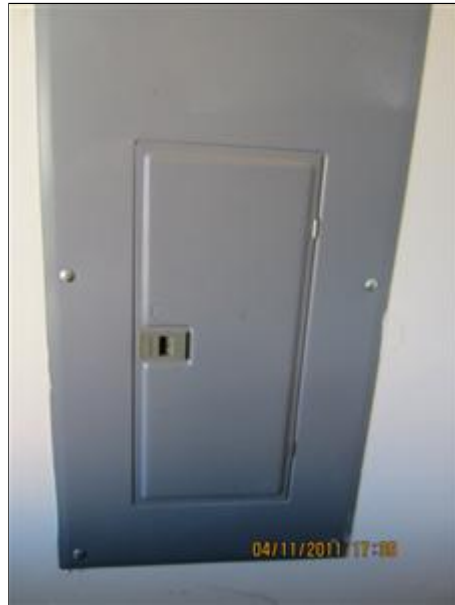
A. Picture 1 Electrical panel
