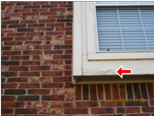
H. Picture 1 Paint peeling and sealant separation
