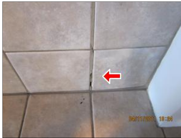
J. Picture 3 Grout cracking in tile
