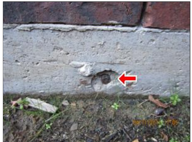
A. Picture 2 Cable end exposed
