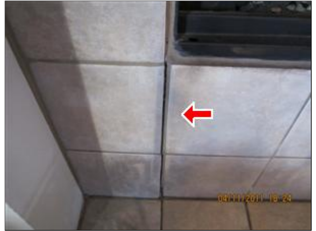
J. Picture 2 Grout cracking in tile
