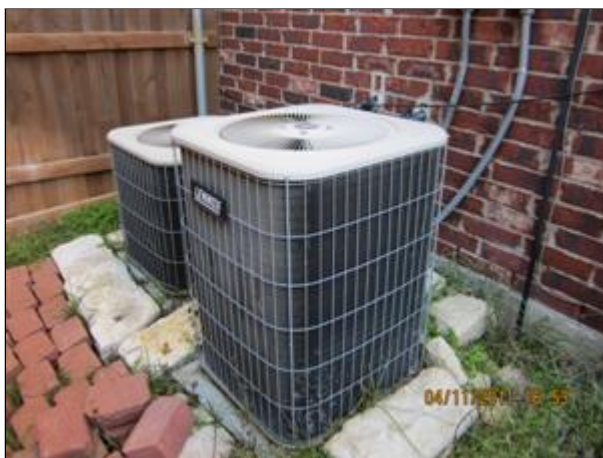
B. Picture 1 Condensing units
