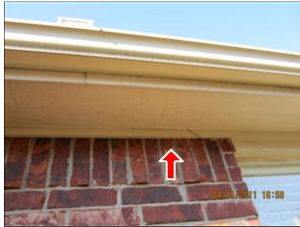
E. Picture 3 Sealant separation
