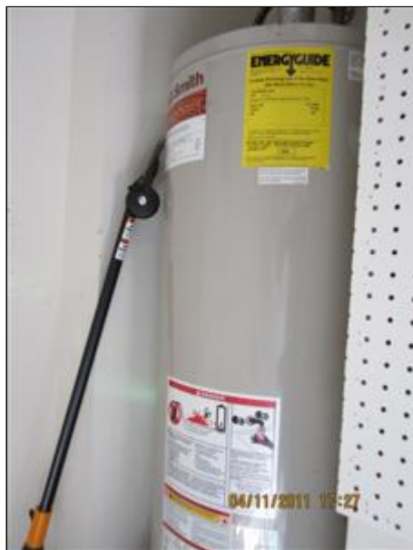
C. Picture 1 Water heater
