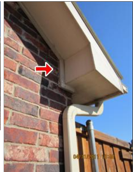
E. Picture 2 Sealant separation
