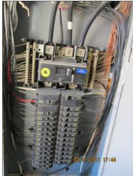
A. Picture 2 Electrical panel
