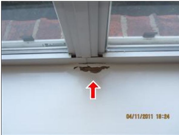
H. Picture 3 Moisture damage to window sill
