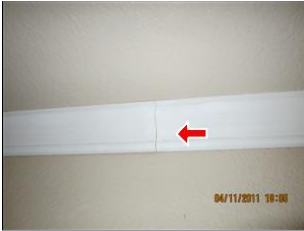
E. Picture 13 Sealant separation at joints in crown mold
