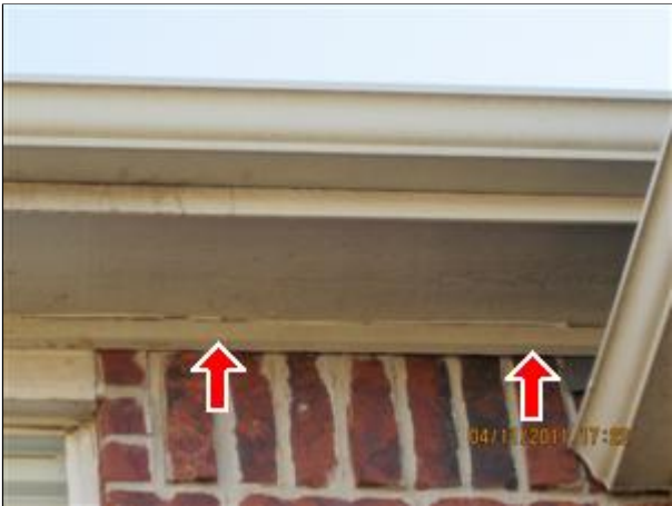
E. Picture 7 Sealant separation
