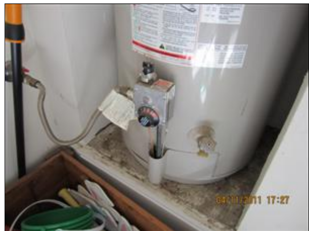
C. Picture 2 No pan under the tank
