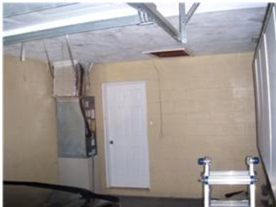
Seal hole where ac condensation line exits south wall.
